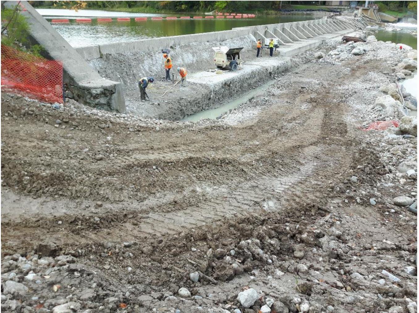
Construction crews working on the rehabilitation of Denny's Dam, an important Sea Lamprey barrier on the Saugeen River, near Southampton, ON. The Great Lakes Fishery Commission is undertaking this project, which began during 2017, in collaboration with the Saugeen Ojibway Nation, Ontario Ministry of Natural Resources and Forestry, and Fisheries and Oceans Canada. Photo: Chris Freiburger, GLFC.
